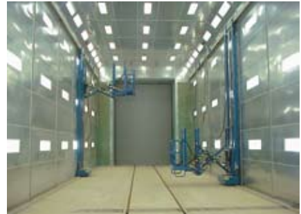
Aircraft Paint Booth: Custom 3-Axis Lift Systems for Painting Aircraft Fuselages
