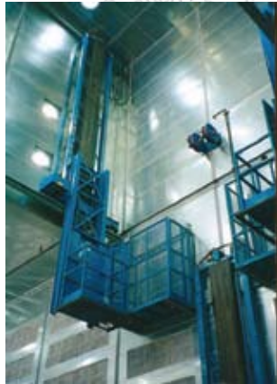
Aircraft Paint Hangar: Custom 3-Axis Lift System to access tail section of aircraft
